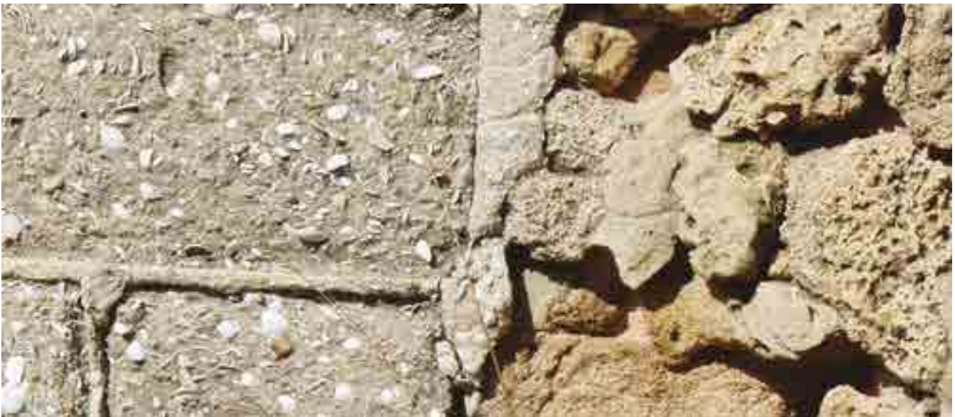
Illustrations 3,4: Remains of an orchard house built in the early 1930s west of the moshava of Ness Ziona: buildings, technologies and building materials. Photo: Irit Amit-Cohen, August 2021
